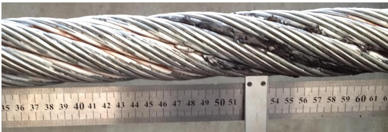
Fig. 1. Formation of dangerous "undulation" factor in the area of steel rope splicing
