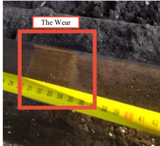
Fig. 9. Wear of the rail as a result of the crane wheel slipping
